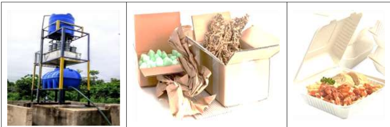
Figure 15: Photos of the INP-HB system installed and the biocomposite products to be produced
